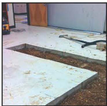
Cutting the concrete floor... A complex trench was built beneath the floor level to provide a delivery method for utilities. The concrete floor was cut and a trough was molded to carry the utilities.
